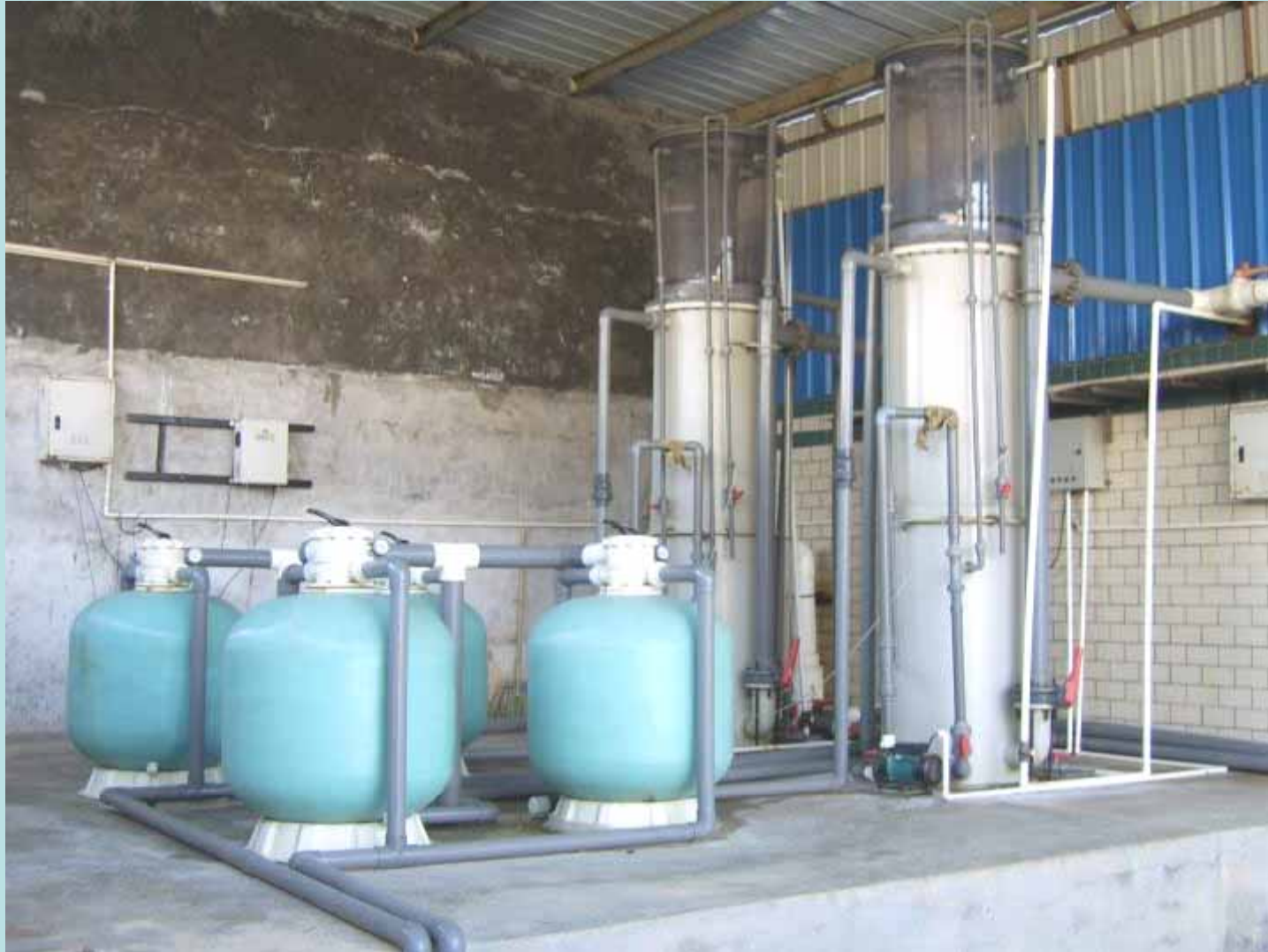
The water treatment system in Evergreen's shrimp hatchery (Sand filters, protein skimmers and ozonators)
