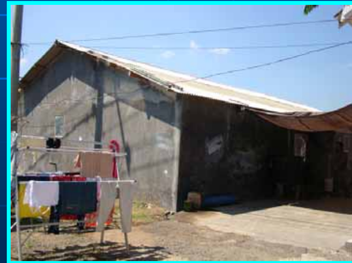
Indoor SBH with cement wall
